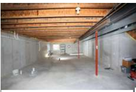
This Shows Only about 2/3 of the Huge Unfinished Basement. So Many Possibilities.
